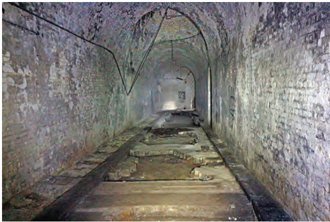
North entrance tunnel; passageway to lower level to right, elliptical air shaft above, the road deck missing many of its wooden blocks. Photo Bob Clary
